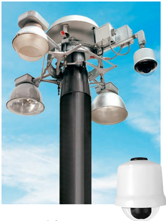
High Mast System HMS® luminaires on lowering device with surveillance camera
